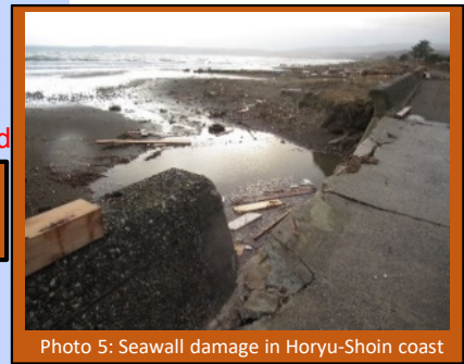
Photo 5: Seawall damage in Horyu-Shoin coast
