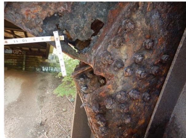
BENT 1, LEFT FRAME LEG, BOTTOM OF THE TOP BRACE Note: areas of severe corrosion and section loss Up to 100%. Typical for Bent 1 Right Frame Leg and Bent 2
