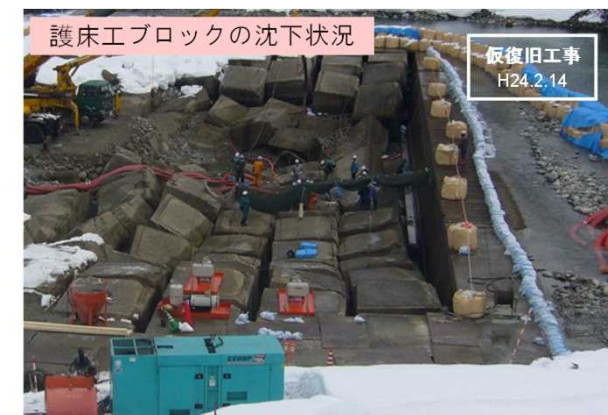
愛本床止め護床工の被災(H23(2011))
